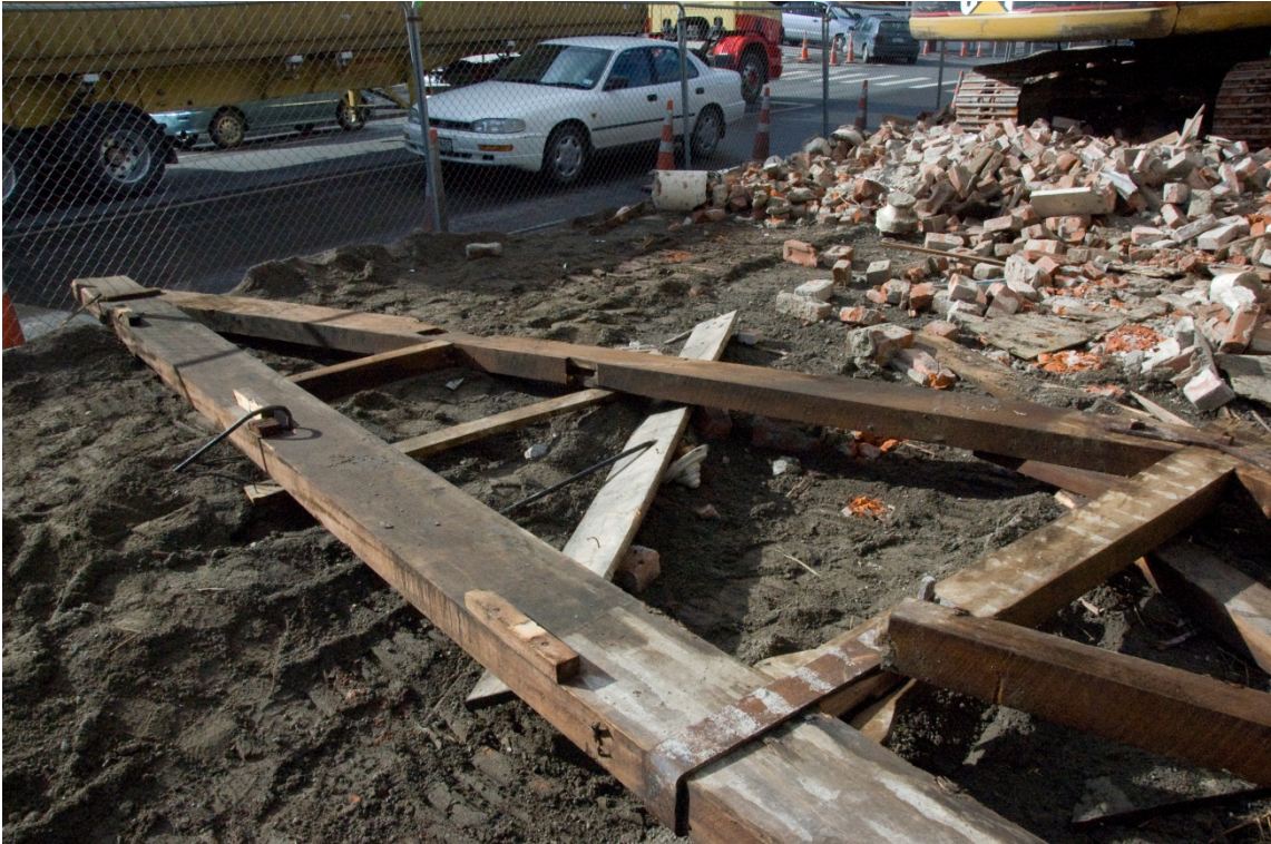
Figure 13. A roof truss, with additional bracing. Note also the staining on the king post, which could be from lath and plaster.
