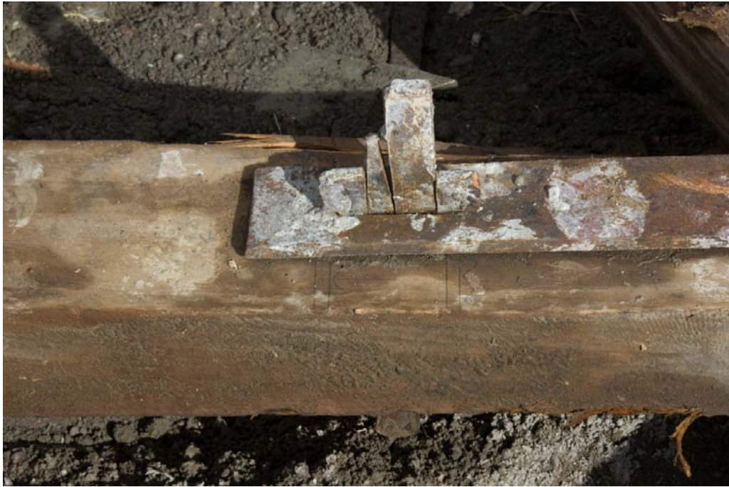
Figure 15. Construction marks and the system of gibs and cotters used to fasten the truss.
