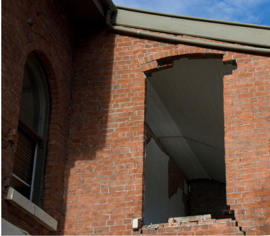
Figure 20. The brick arches on the first floor of the west elevation (left) and the lean-to (right).
