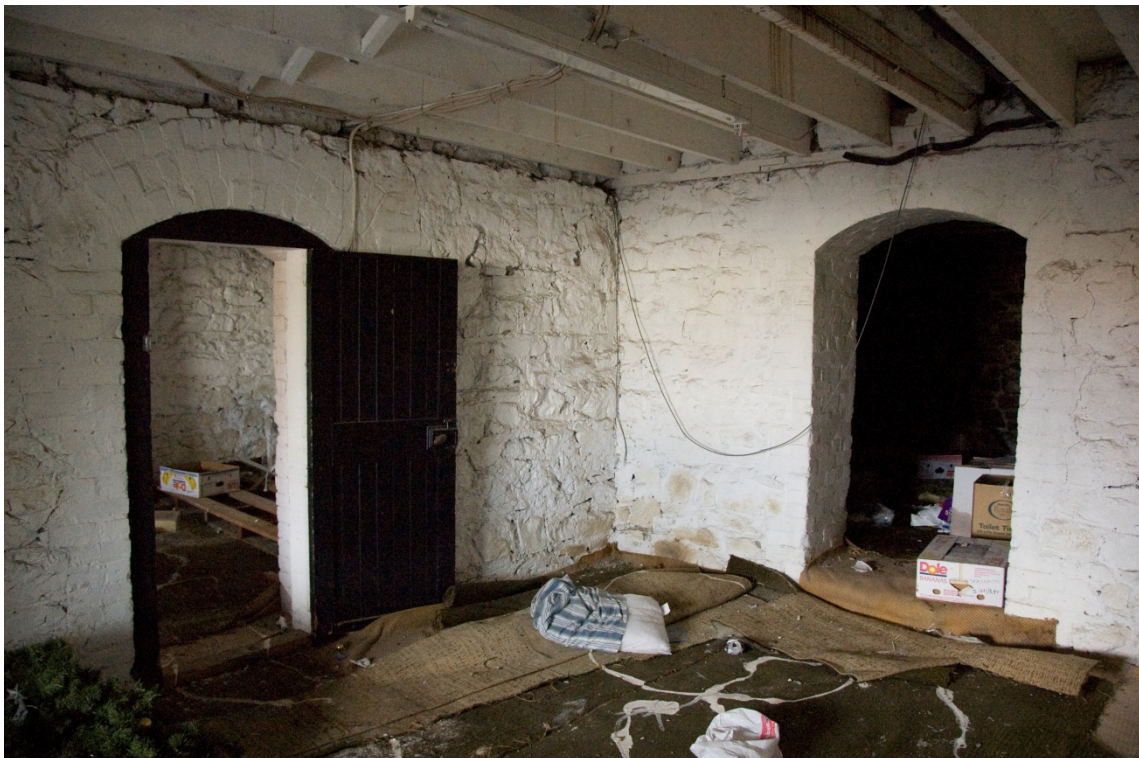
Figure 18. The basement, showing the form of the ground floor above. Note also the form of the arches above the doors.
