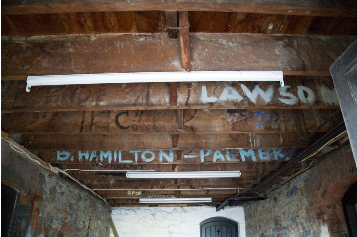
Figure 33. Graffiti on the ceiling of the basement.
