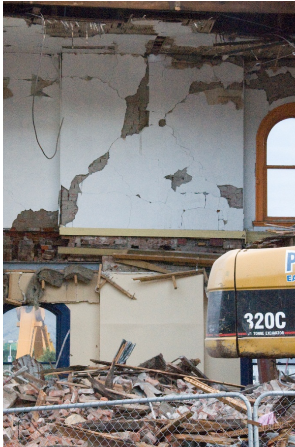
Figure 42. The ground and first floor fireplaces on the south wall of the building. Note the width of the first fireplace in relation to that on the ground floor.
