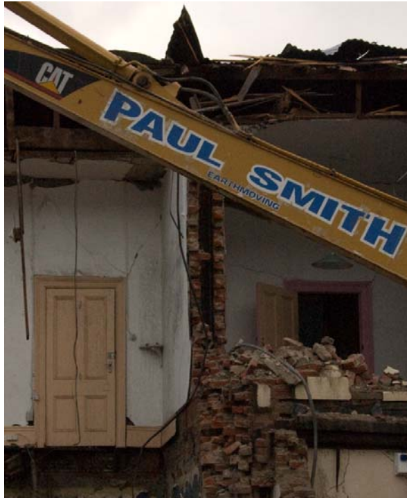
Figure 11. An interior wall on the first floor, showing a cavity that was probably related to the air flues used to ventilate the building.
