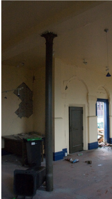
Figure 17. A metal column supporting an I-beam (the casing around the I-beam is visible) on the ground floor.
