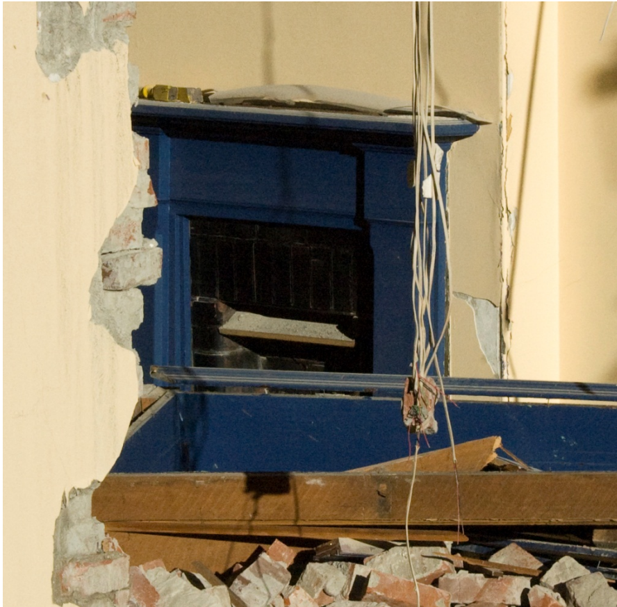
Figure 39. The fireplace in the room to the south of the office. This did not have a coal register but the form of the fire surround was the same as that in the restaurant.
